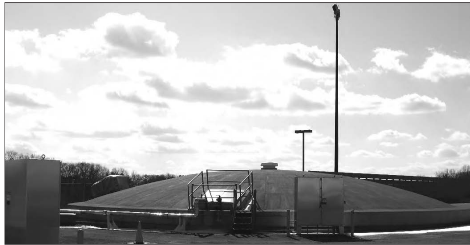
All glycol contaminated fluid collected at Bradley is deposited to two, one-million gallon underground storage tanks. From these storage tanks, the material is piped to Inland Technologies' plant for recycling.
