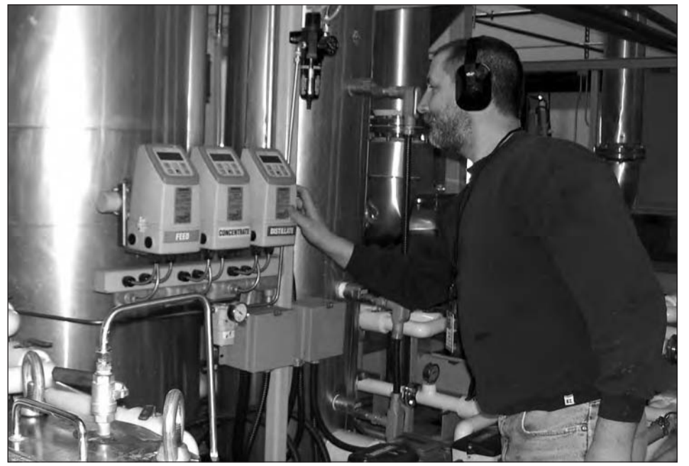
A technician runs a system check on Inland's Glycol Concentrator at Bradley. This patented system uses about one-tenth the energy of traditional distillation systems to separate water from the waste chemical.
