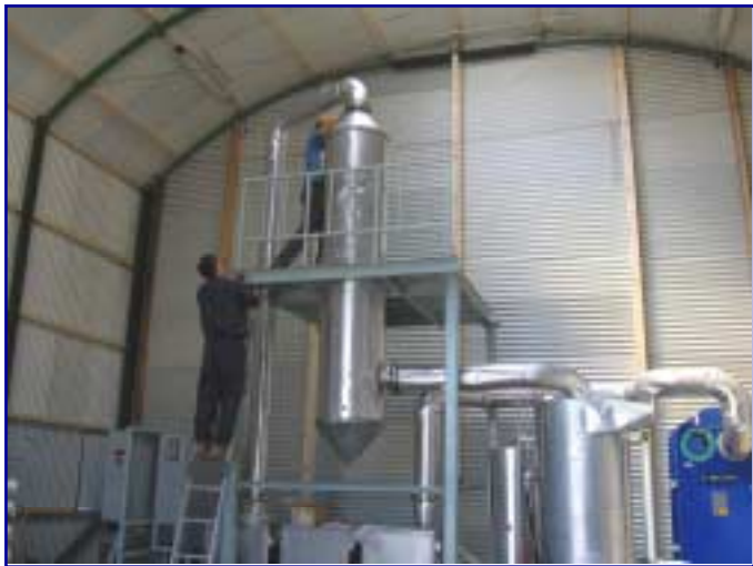
Commissioning of the Glycol Concentrator at Schiphol. The unit can process about five million liters of glycol effluent in a year.
