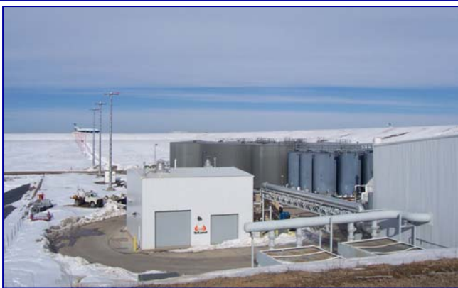
Outside view of the glycol recycling plant at Denver Airport. The site hosts Inland's Glycol Concentrator's, the airport-owned distillation plant [operated by Inland] and the tank farm.
